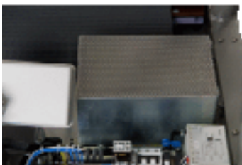
Frequency inverter metal housing (for shielding)
