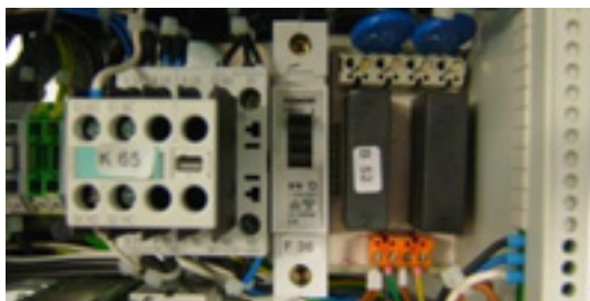
Secondary fuse isolation transformer 1-pole B16A
