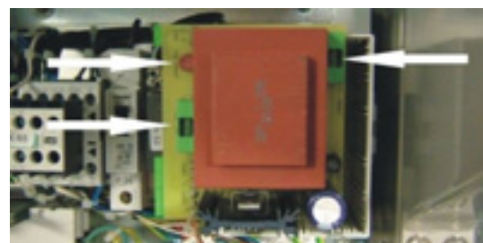
Fuses in cabinet for power supply unit
